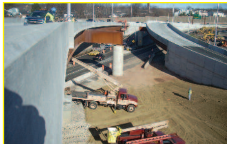
Overhead ramps B and SE at Interchange 142 (photos courtesy of Gannett Fleming)
